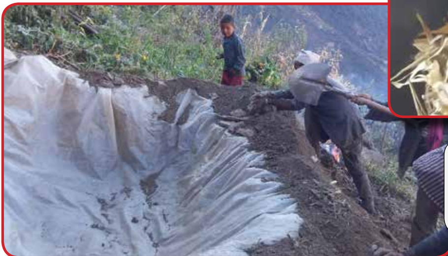
Left - Residents of Bhadaura complete a water tank for small scale irrigation to kitchen gardens and fruit nurseries in their village.
